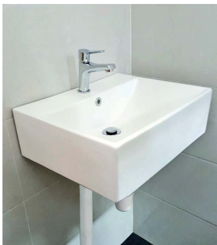
Wash basin with tap mixer
